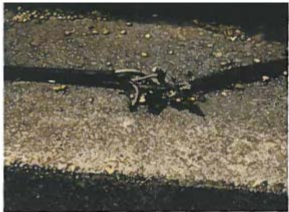
4. Damaged Electrical Cord Identified in 2008 Insurance
