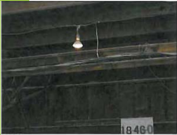
3. Exposed 440-Volt Electrical Wiring Identified in 2007 Survey
